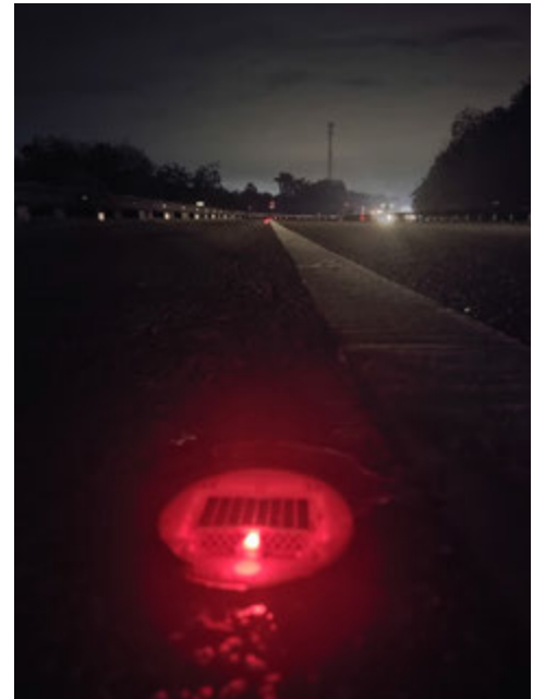
Red SOLARLITE road stud embedded along the slow lane side of the NSE
