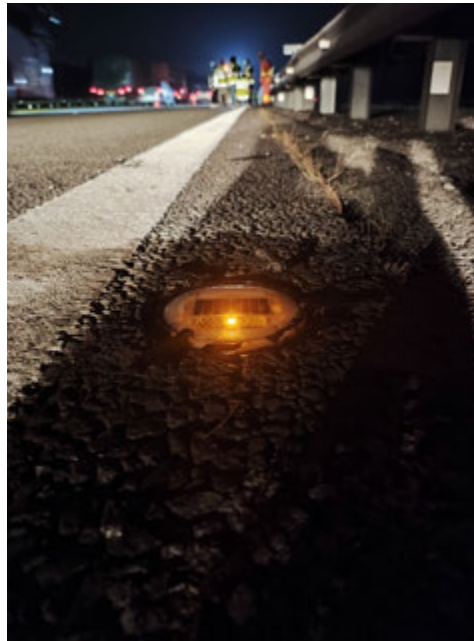
Amber SOLARLITE road stud embedded on the fast lane side of the NSE
