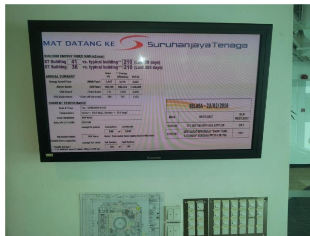
Figure 4: Display screen of the energy management system
