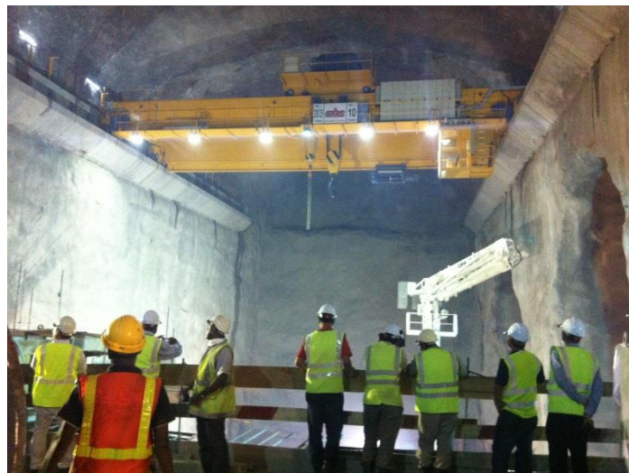
Underground Power House
