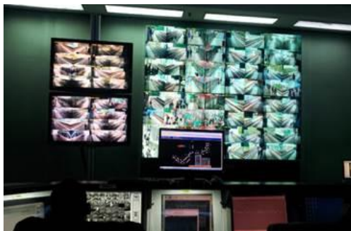
Operation control room
