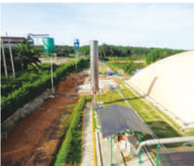
BIOGAS PROJECT-METHANE GAS CAPTURING
