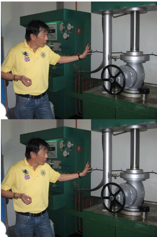
Mr. Lim showed how the valve been tested
