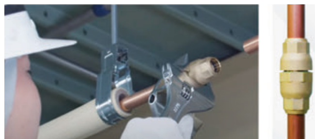
Figure 6: Braze-less piping eliminates open flames and copper-oxide contamination risks, simplifying permits and improving compressor/expansion valve health
