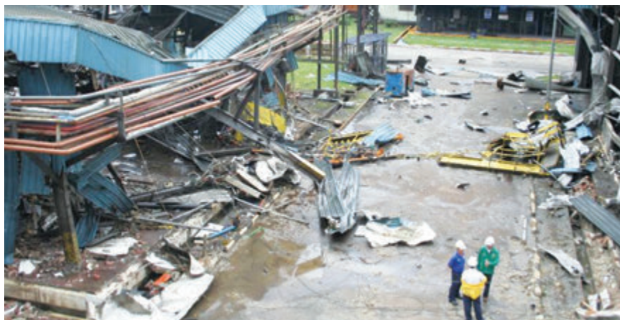
A damaged boiler house after a boiler explosion occurred
