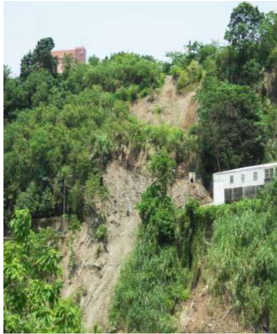
Figure 1: Multi-tier reinforced slope failure in Taichung, Taiwan on 1 st Sept 2013
