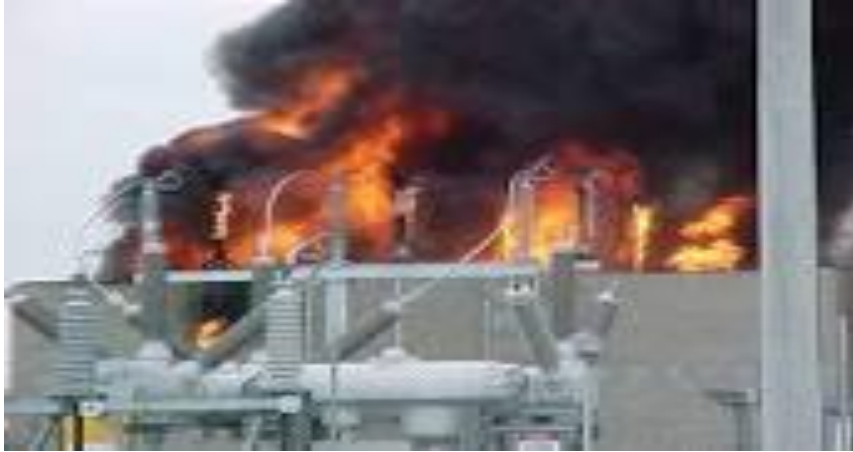
Typical Power Transformer Fire
