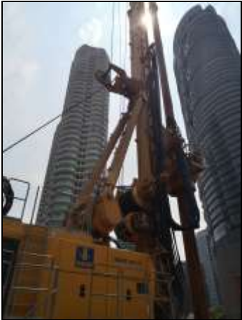
Figure 1: World’s biggest boring rig Bauer BG 72 specially customised to suit project specification for bored pile construction works
