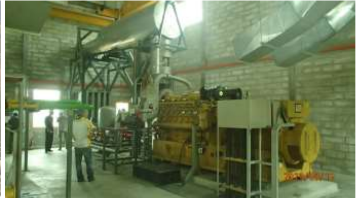
Biogas power house- power generator- Gas engine
