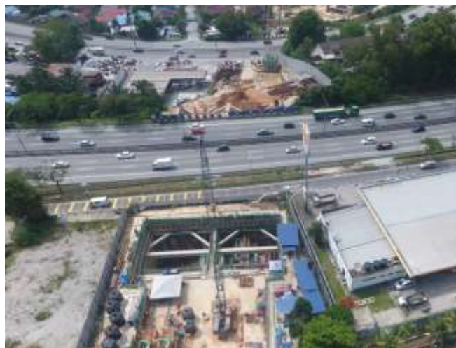
Figure 1: Bird's-eye view of the tunnelling worksite beside KL-Seremban Highway near Kuchai Lama
