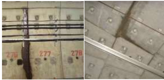
Figure 3: Typical leakage at concrete lining joints of metro tunnels in Shanghai
