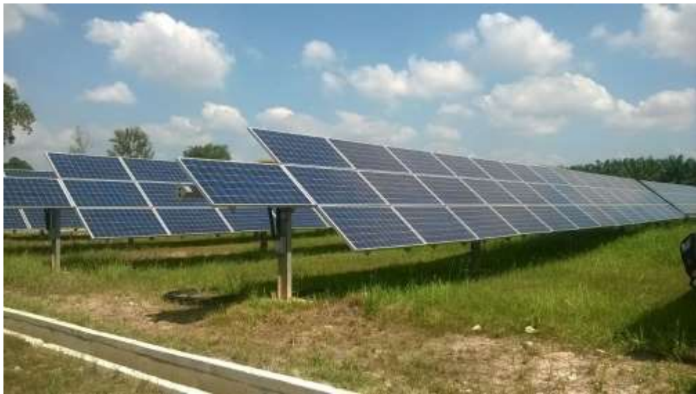
Some of the installed solar panels
