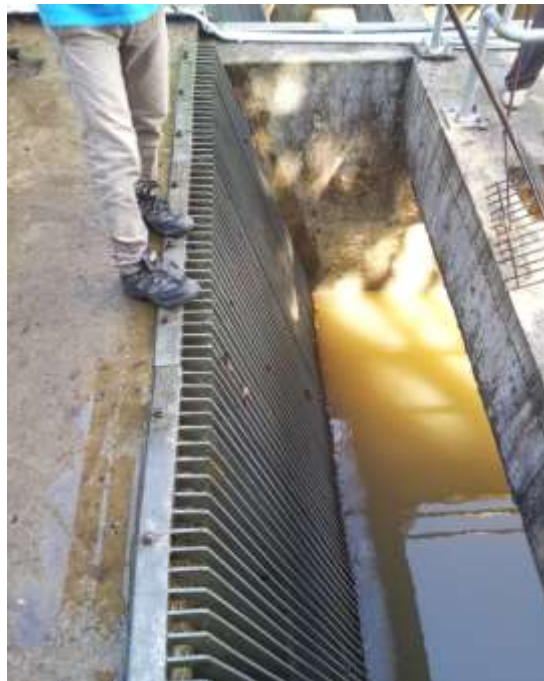
Figure 4: Trash rack for filtration purpose
