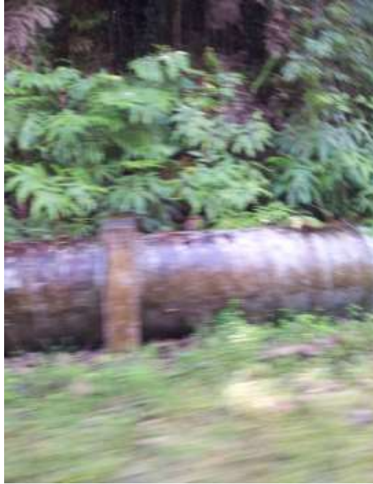
Figure 3: Pipe to transfer water to the powerhouse
