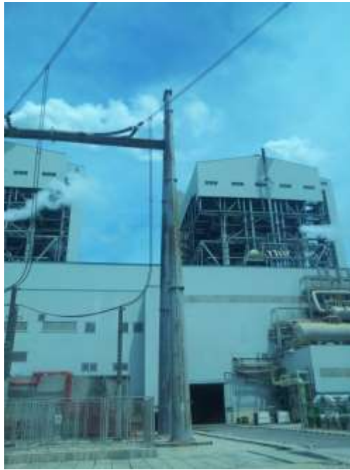
Figure 3: Once, the largest transformer in Peninsular Malaysia
