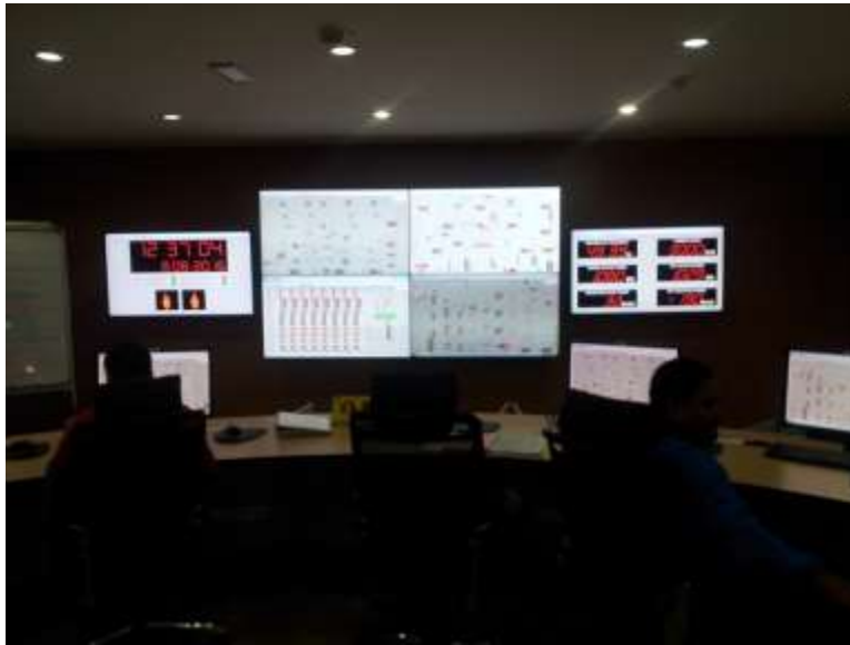
Figure 1: Simulator room to train the staff on monitoring work
