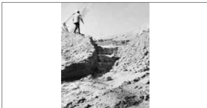
Figure 7: Dubai Dry Dock – rapid erosion of the downstream face of the bund.
