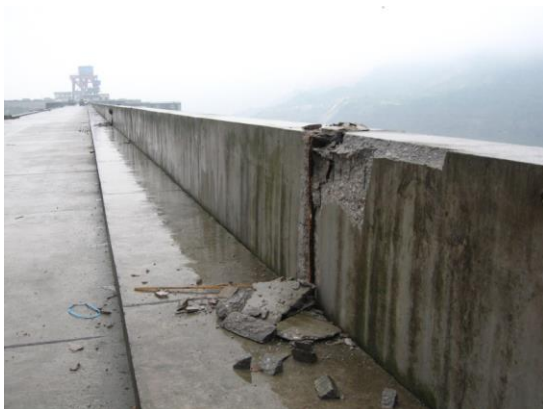
Rupture of Wave Wall after Earthquake
