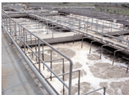
Figure 5 : Aeration Tank with Diffused Aeration System
