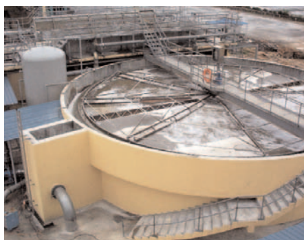
Figure 3 : Dissolved Air Flotation Clarifier
