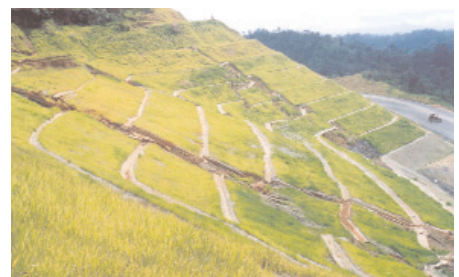
Slope failure in graphitic schist - Lojing highway
