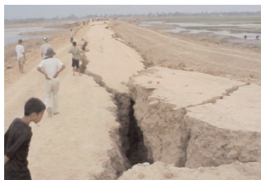
Typical fracture of a rural road due to instability of the underlying soil
