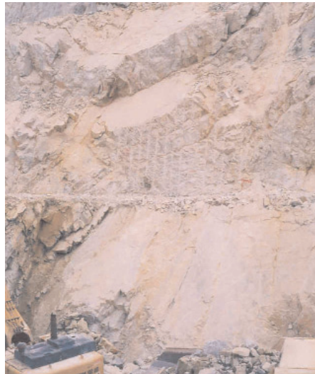
Plane failure in granite rock slope - SILK highway
