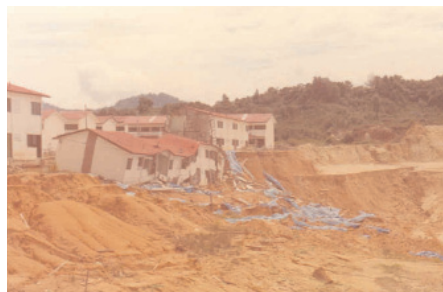
Slope failure in ex-mining land due to rapid draw-down phenomenon : Cheras, K.L.
