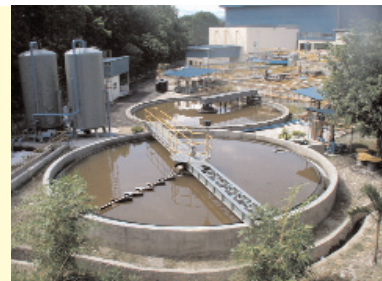
Figure 6 : MMF and Secondary Clarifier
