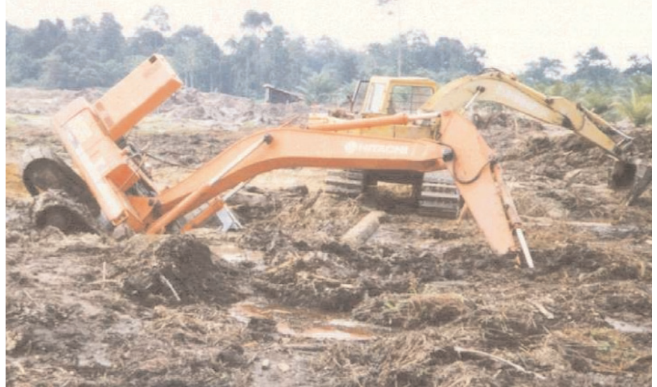
Problems arising from construction over soft soils area commonly solved by installing geosynthetics directly over the soft subgrade
