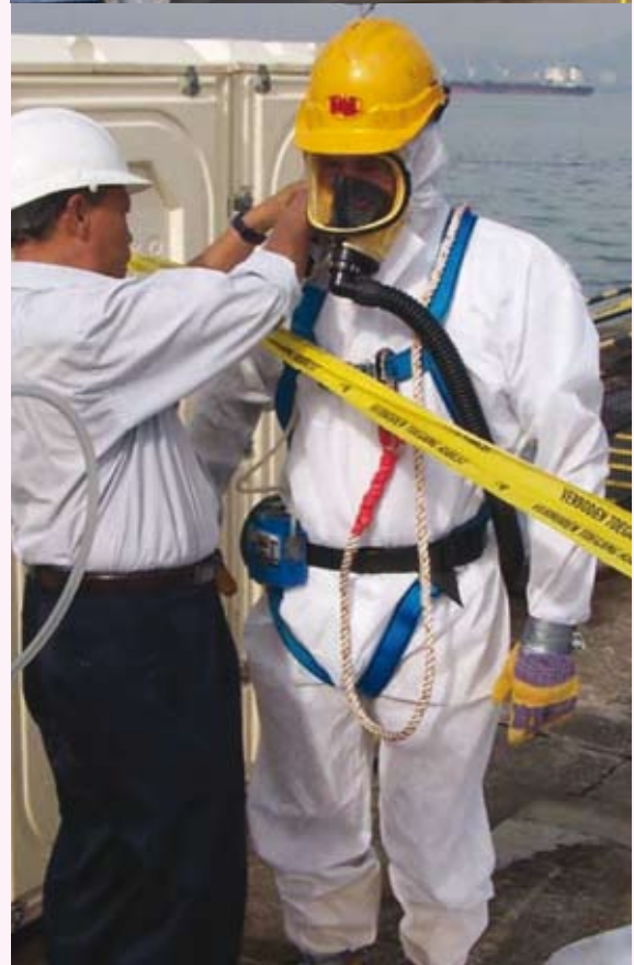
Asbestos removal personnel removing asbestos roof sheet from one of the multi-national company in an oil terminal. [Courtesy of TMR-DDM Demontage Sdn Bhd]
