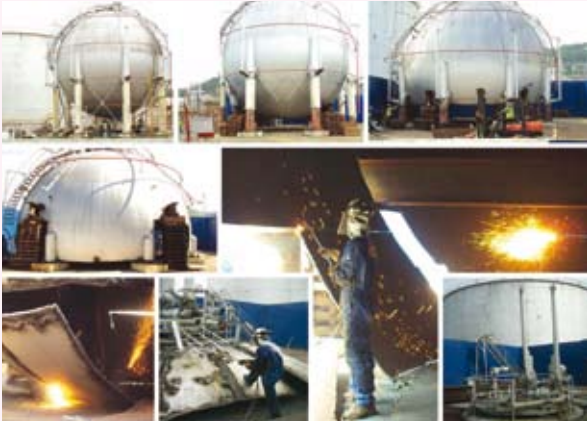
Controlled demolition of LPG Spherical Tank in one of the multinational company in an oil terminal. [Courtesy of TMR-DDM Demontage Sdn Bhd]
